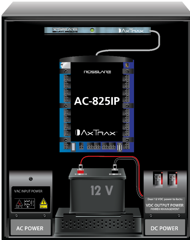
Figure 14: AC-825IP in the ME-1515 Enclosure
