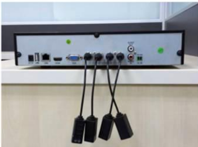
Old baluns make the cabinet a mess
