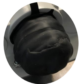
Wrap another layer of rubber mastic tape all over the Ethernet port
